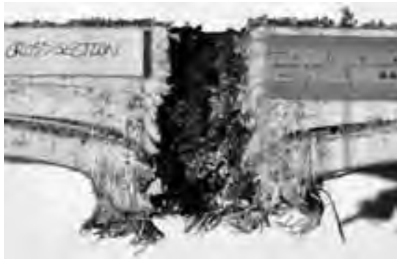
Figure 27: F5 – S2 Liner Deformation
