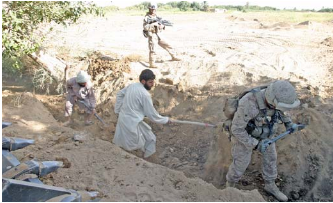
Image 8: Sgt. Cody T. Romriell, a combat engineer with 2nd Battalion, 9th Marines, helps local farmers dig out a clogged canal during the construction of Typhoon 3 in Marja, Afghanistan, Sep. 9. Marine engineers with 2/9 have been constructing new patrol bases in their area of operation in order to increase force protection. Typhoon 3 is one of the many being built.
