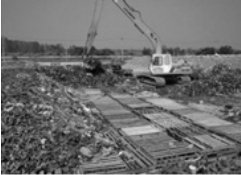
Figure 3.2 Mechanical biological treatment prior to landfill in Phitsanulok Thailand (Photo: Suthi Hantrakul)
