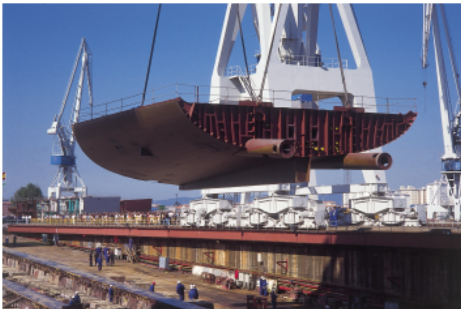
Fitting the keel of the Álvaro de Bazán F-101 frigate at the Bazán factory in El Ferrol, June 1999.
