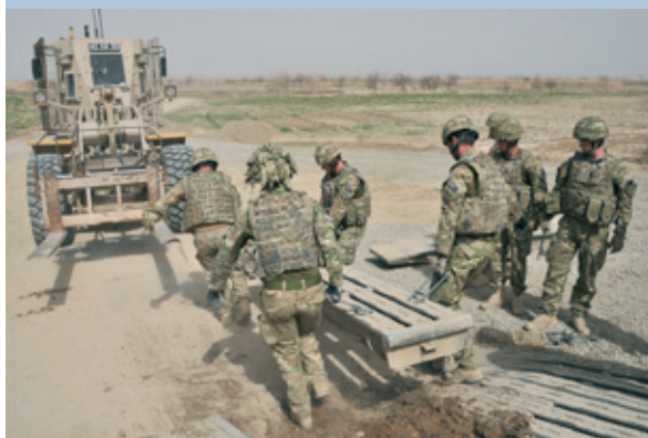
Royal Engineers from 37 (Three Seven) Squadron strip a Medium Girder Bridge (MGB) near Check Point Oqob in the northern part of Nahr-e Seraj District of Helmand Province.
