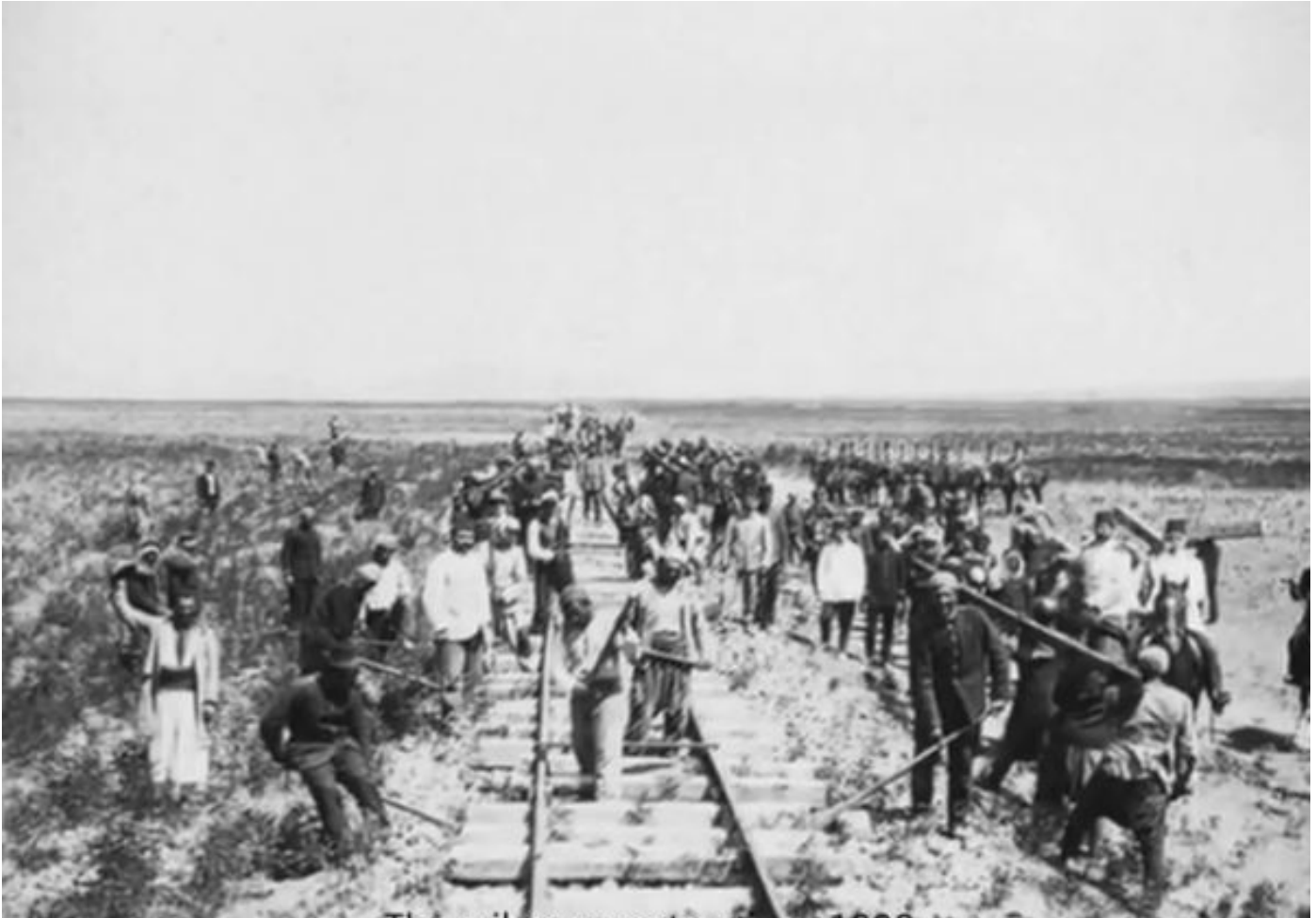
1890. Constructing the Jaffa-Jerusalem railroad. Workers were brought in from Egypt, Sudan, and Algeria.
