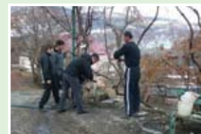
Community members in Buzal turn on the tap after successfully laying a pipe to bring water to the village, Dzhava district, May 2012.
