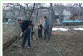
Community members lay plastic piping to bring water to Buzal community, Dzhava district, May 2012.
