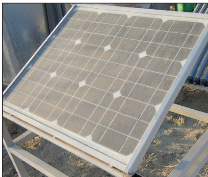
Fig. 10: Samples of dirty PV panels because of accumulated dust deposition
