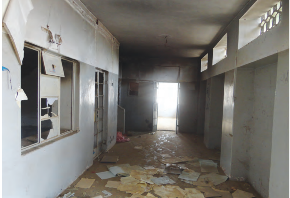
Photo 3. Primary court in Zinjabar, Abyan, after damage and looting in the 2011 conflict
