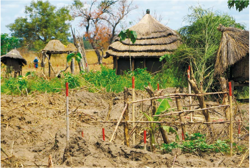
A MineTech International demining site in Kuda with suspected AVM presence. The red posts indicate boundaries marking mine presence.
