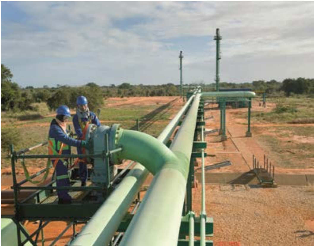
SASOL gas pipeline in Temane, Mozambique
