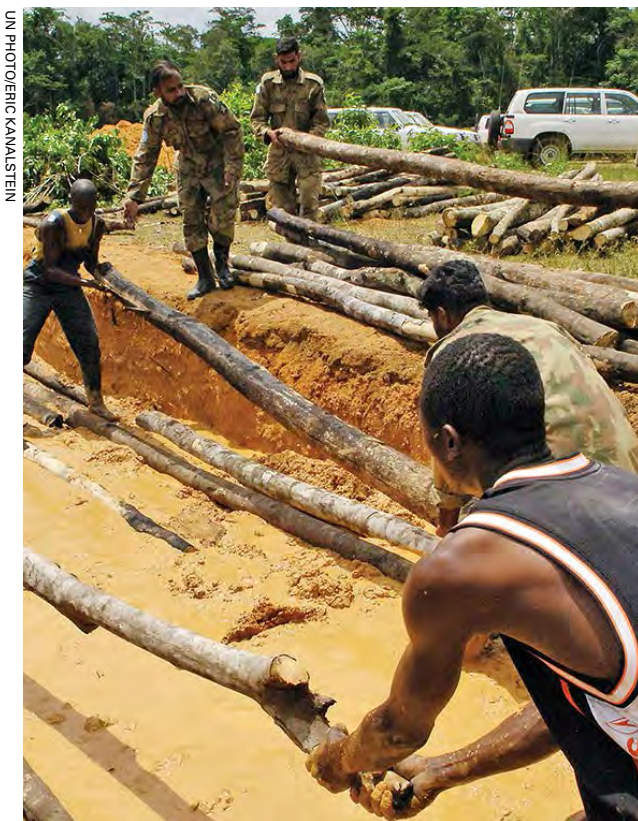
United Nations Mission in Liberia (UNMIL) peacekeepers and Liberian villagers repair a flooded road on the outskirts of Voinjama, Liberia (April 2006).
