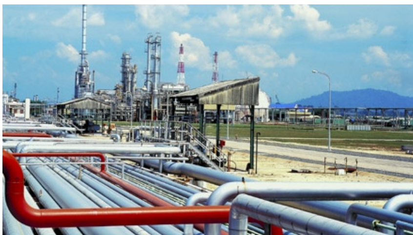
An oil refinery in Malaysia
